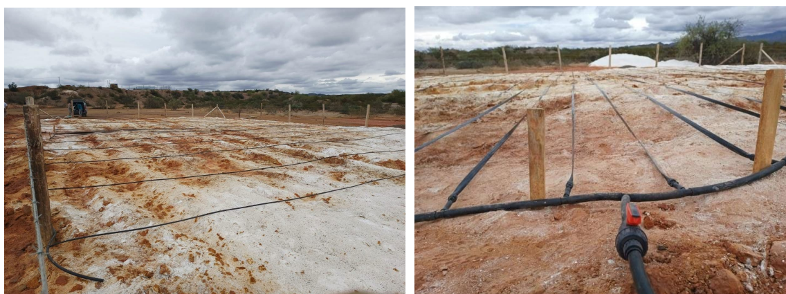
Figure 7-5. Irrigation system installed in experimental plots
