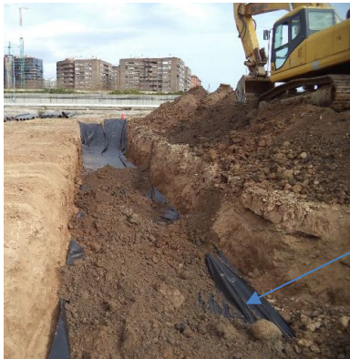
PEAD geotextile fabric installed to prevent contaminant leaching to non-impacted soil layers
