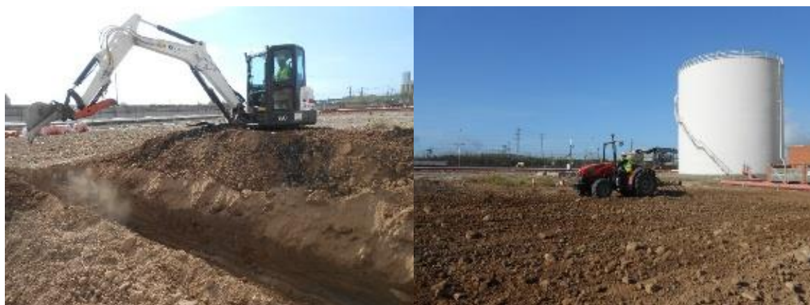
Figure 4.1 Excavation works aiming to have TPH contamination in the upper layers (left) and tilling activities (right) performed prior to the second growing season of Sorghum
